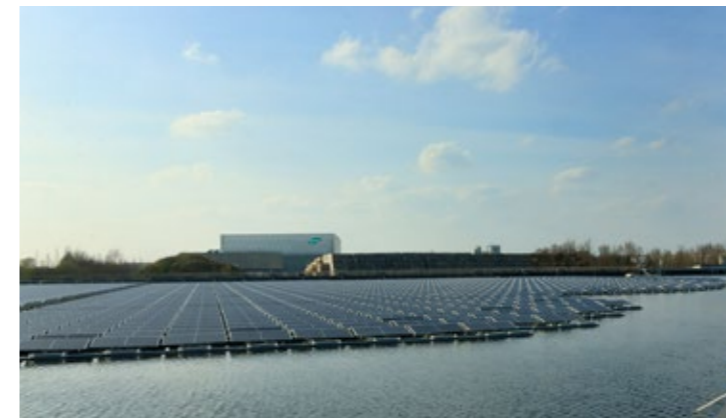
Irrigation bassin with solar pannels
